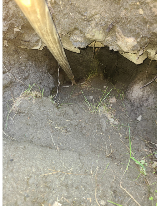
Figure 3 – Lower Sinkhole Section
