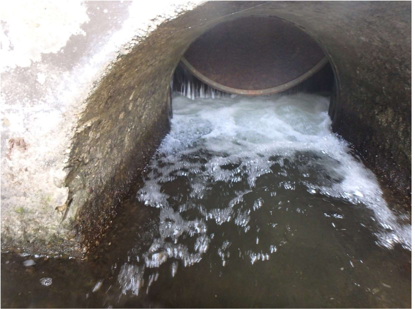
Photo 3: The gate plate extending into the 36 inch concrete pipe waterway opening. From the invert of the pipe to the bottom of the plate was measured to be approximately 21 inches. From the bottom of the plate to the crown of the pipe was measured to be approximately 15 inches.
