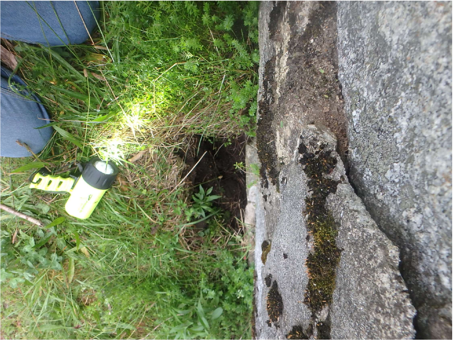
Photo 2: Small sinkhole upstream of the stone masonry wall near the existing sinkhole.
