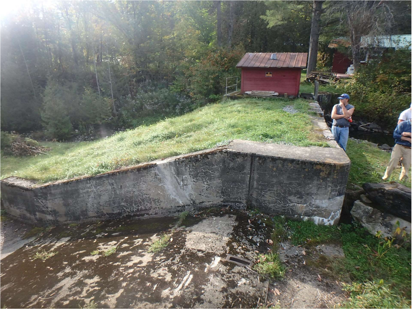
Photo 1: The dam from the auxiliary spillway looking at the gatehouse. The temporary sinkhole repair on the crest can be seen.
